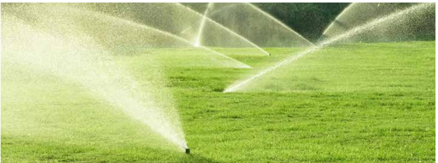
Automatic garden sprinkling system
